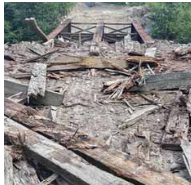
The demolished bridge on the only road out of the area left cottagers stranded.
